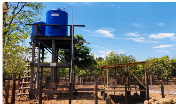
Water Connection System (Water Solar Pump)
